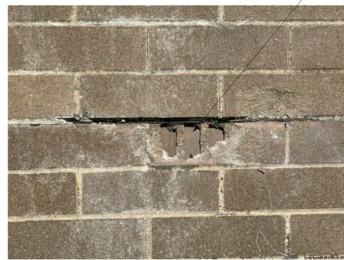
2 (E) SPALLED BRICK, TYPICAL
