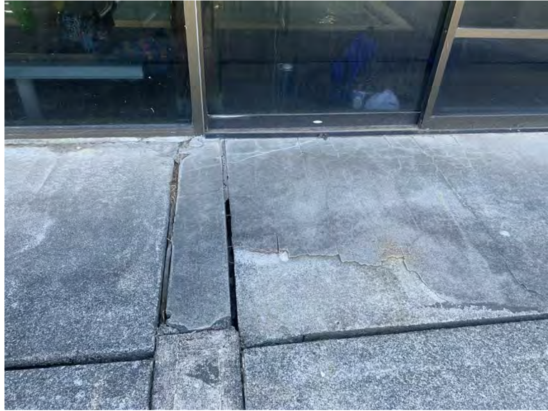
1 (E) CRACKED CONCRETE @ (E) SIDEWALK
