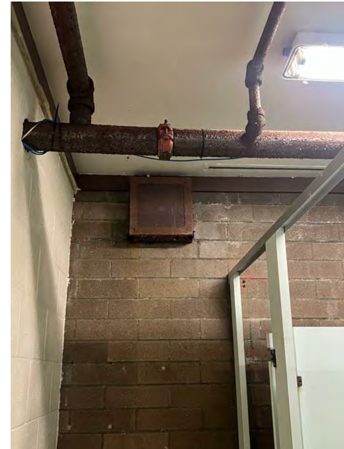
18 (E) CORRODED PLUMBING PIPES 1/4" = 1'-0"
